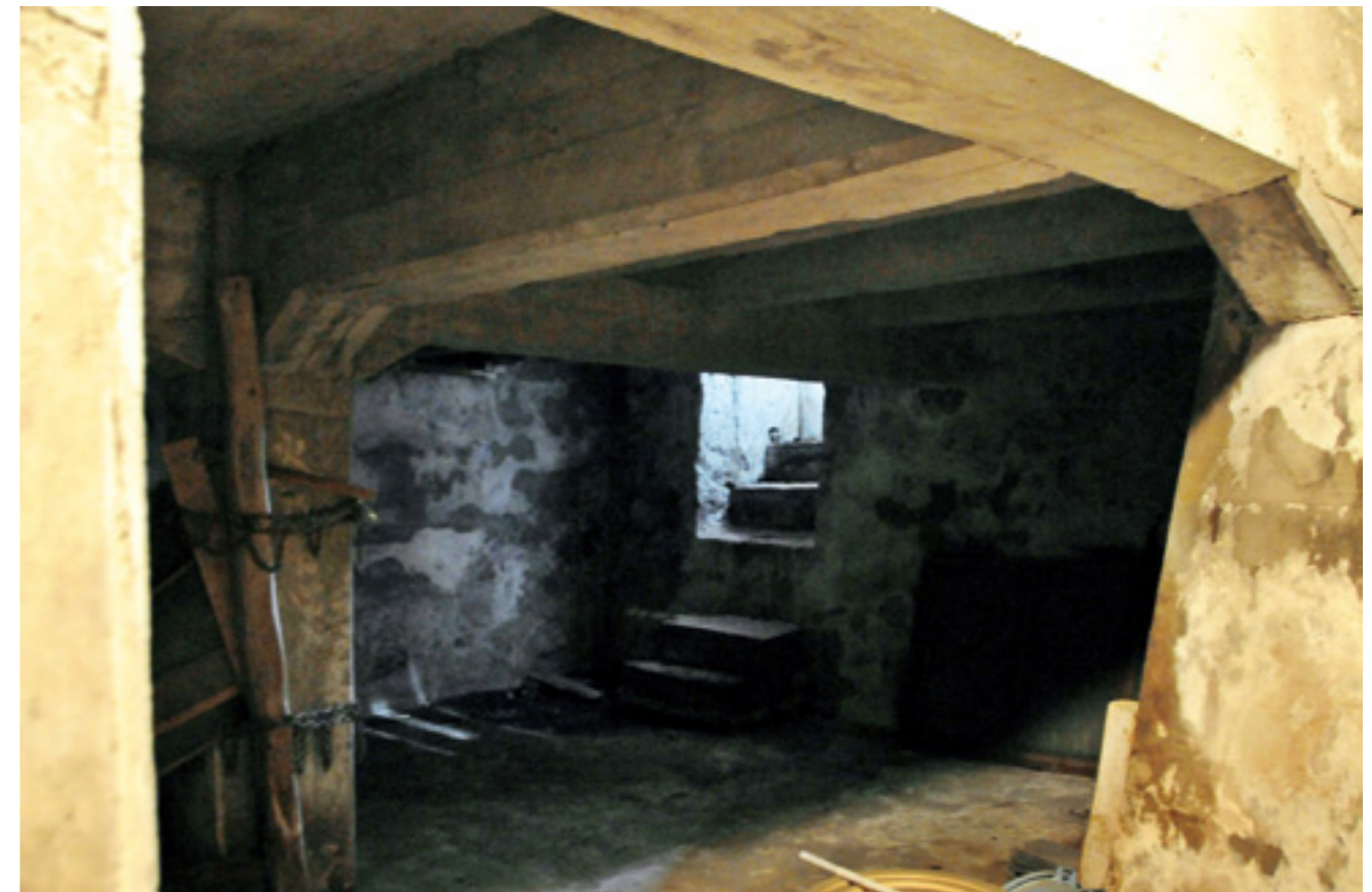
↑ The basement room of a mercantile house near Tarumi-ya. The whole place is now covered by mortar walls. The horizontal tunnel at the back is a stone staircase that makes good use of the geographical terrain. However, it could not be ascertained if this had been an underground chapel.
